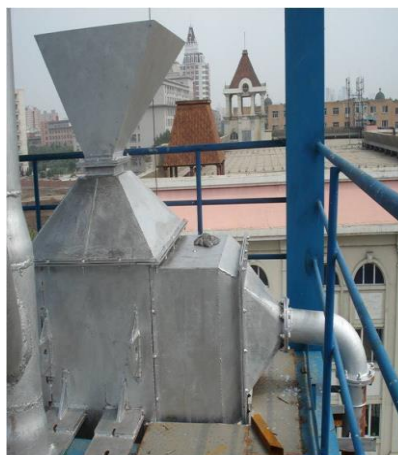
Figure 6. The Real High-speed Compound Heating Furnace
