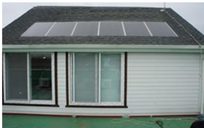
Figure 7. View of the Roof-Integrated PVT (BIPVT) on the Experimental House
