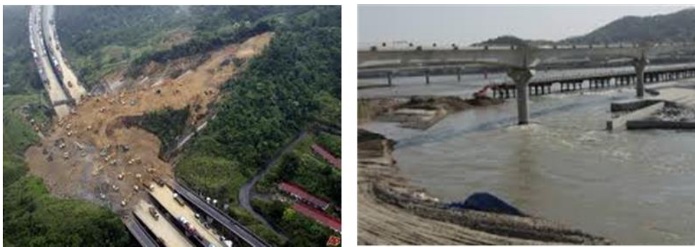
Figure 1. Damages to a Road and Bridge
