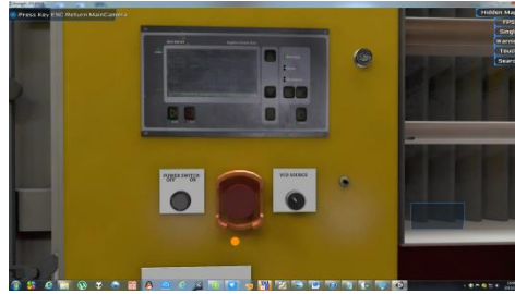
Figure 23. Local Control Box
