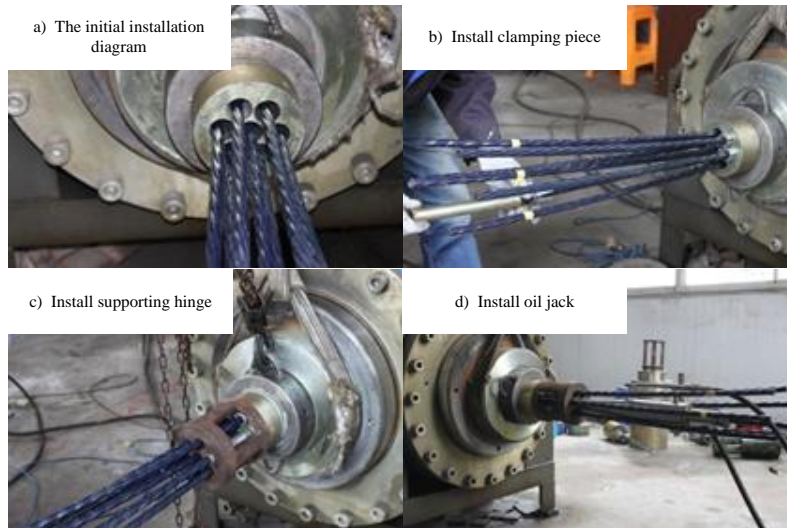
Figure 7. The Installation Process about Oil Jack and Clamping Piece Next Anchor Plate
