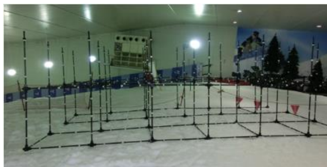
Figure 2. A View of the Control Boxes Installed
